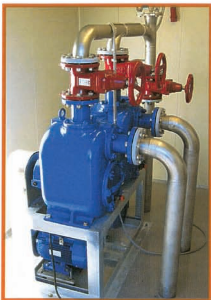
Sewage Lift Station
