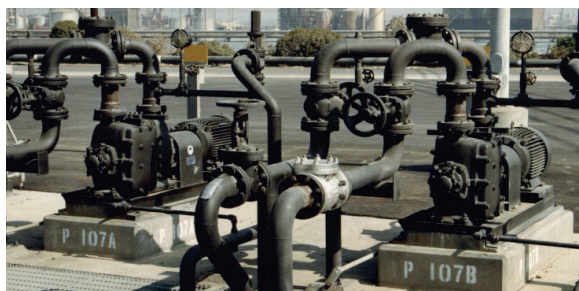
▲ Two L400 pumps, pumping wastewater at an oil refinery
