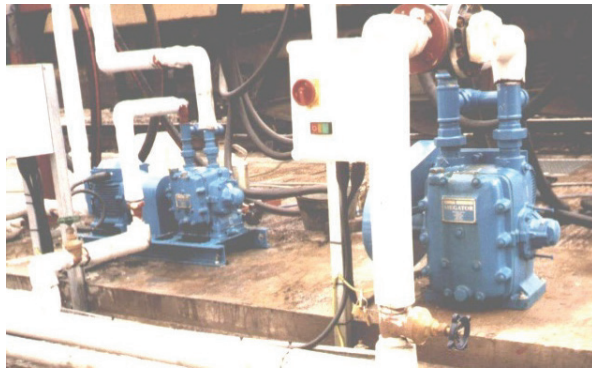
▲ Pumping diesel fuel to a railway locomotive
