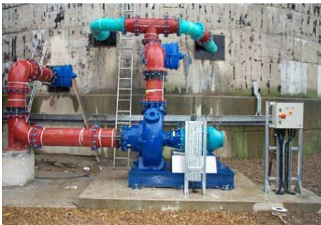
Twin Nozzle Systems Mixing Sludge stored in a 3,200m 3 Storage Tank
