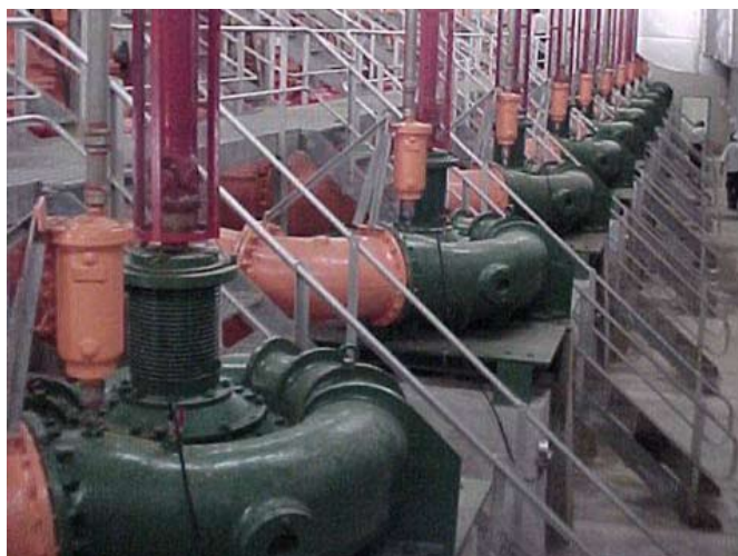
10 off L20K [500 mm] inlet pumps. Duty 980 l/s @ 24 m
