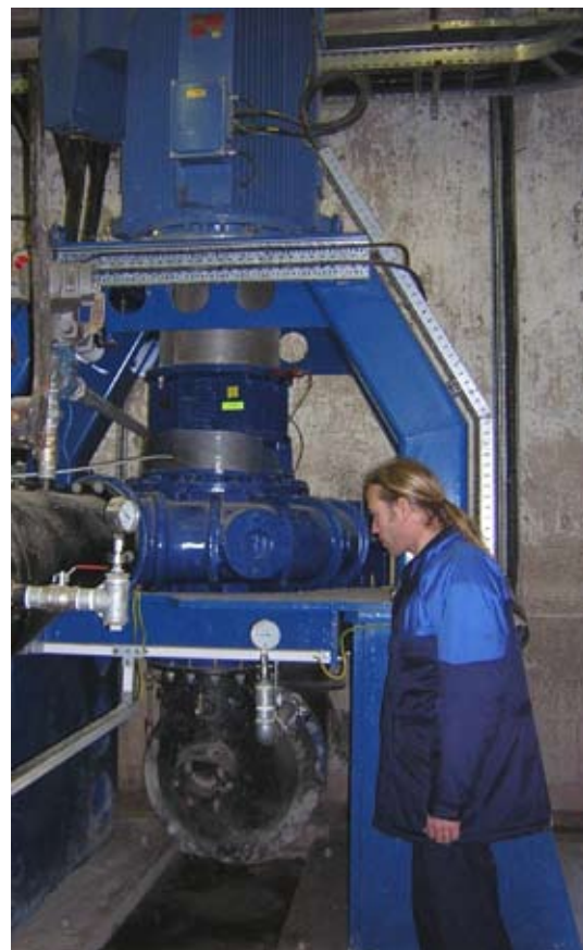
2 off FO mounted 400 kw pumps handling unscreened raw sewage
