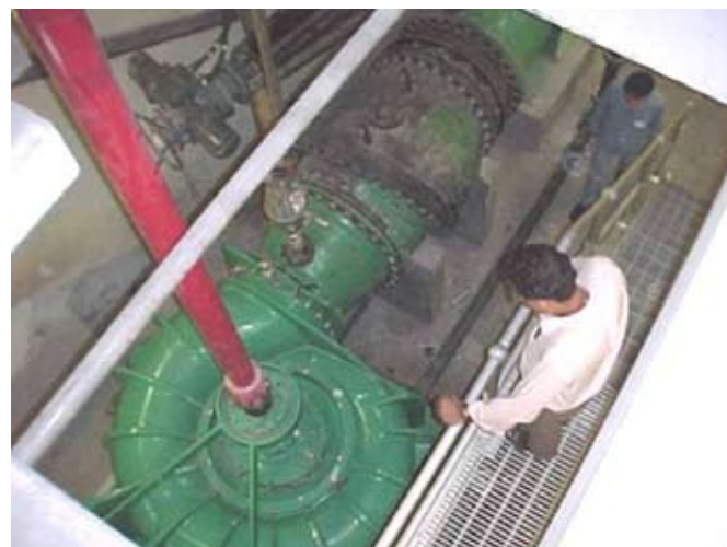
M28K [700 mm] raw sewage pump with 500 ks motor. Duty 1500 l/s @ 25 m
