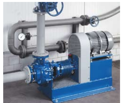
A horizontally mounted belt driven pump
