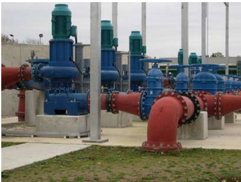
6 off BO mounted 250 mm pump handling RAS
