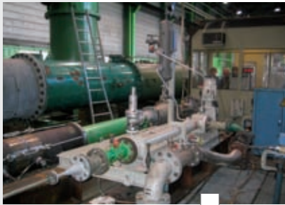
Flare knockout drum, Middle East
