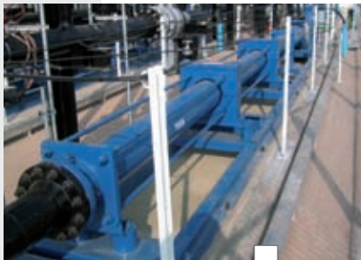
Multiphase booster, Thailand
