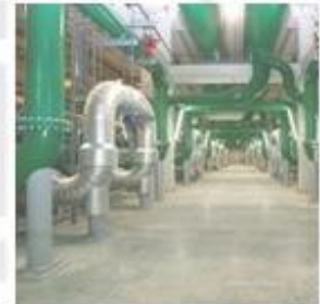
Cooling water systems
